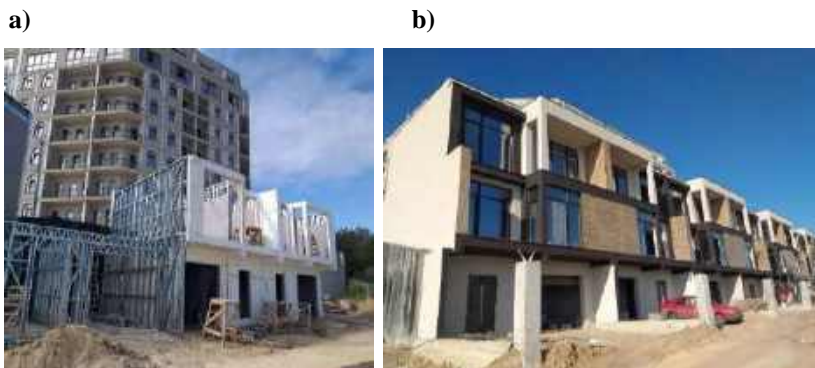
Fig. 3 – Example of the use of the patented technology of frame permanent formwork UA 154847 «Frame permanent formwork system» during the construction of townhouses on the Black Sea coast in Odesa. The external cladding of the frame is made of polystyrene, and the internal cladding consists of two layers of moisture-resistant gypsum board: a) – the process of constructing enclosure structures for the townhouses; b) – general view of the completed townhouses
