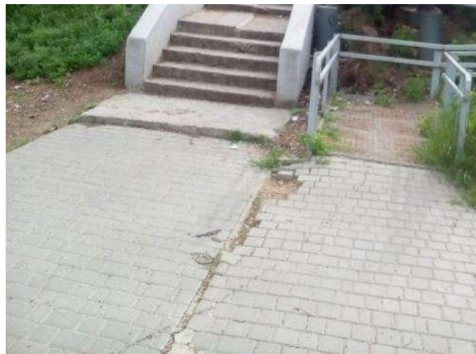
Fig. 4. Destroyed part of the newly-paved footpath near the ramp
